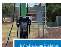
EV Charging Stations
